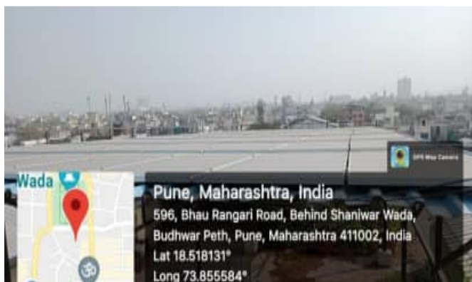
Photograph of 20 kWp Roof Top Solar PV Plant:
